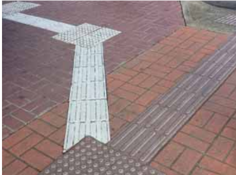
existing conditions of pavement within village
