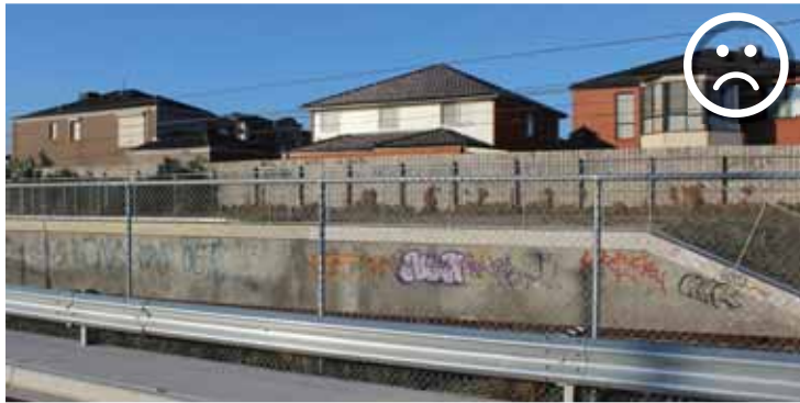
poor retaining wall response adjacent to residential land
